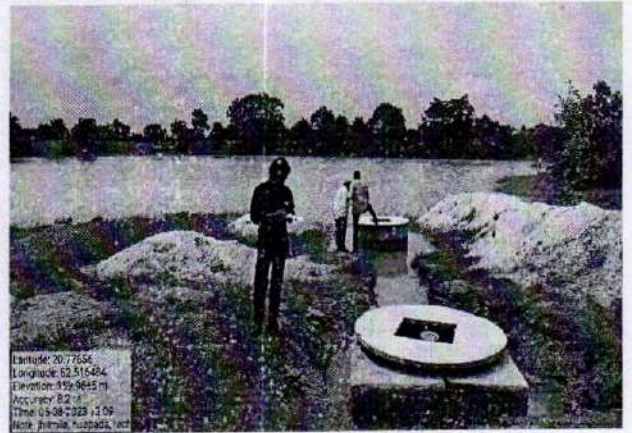
Percolation Ponds with Recharge Wells
